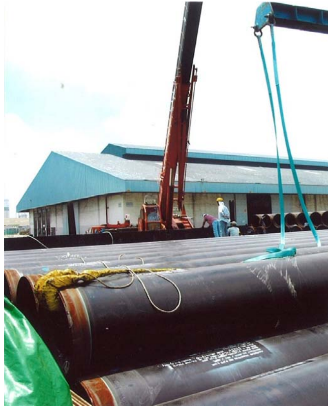
Unloading the Coated Pipes from our Barge in Jurong Port The collection was done in Batam
