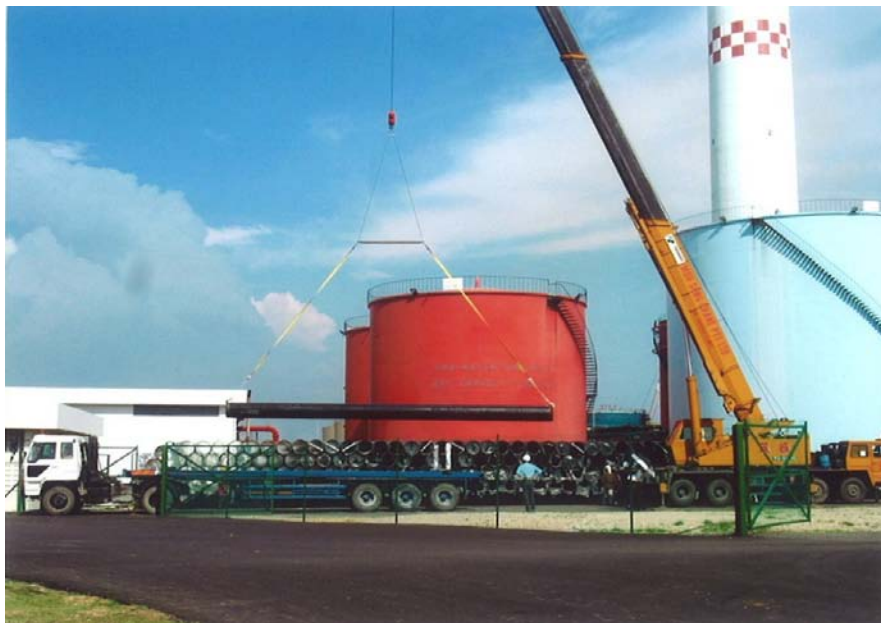
Offloading and Stacking the Coated Pipes in the open storage inside Tuas Power Station
